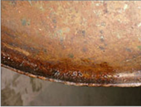
A leaky seam
