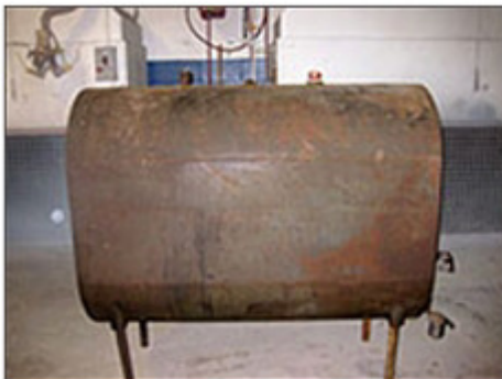
A Bad tank. Notice the seeping along the bottom
